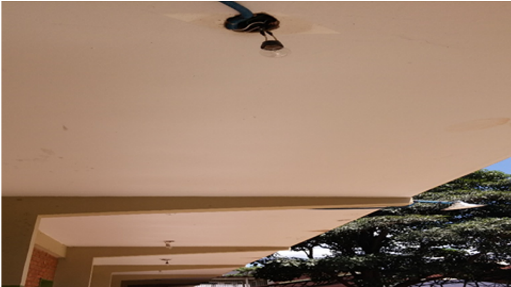
Photograph 2. Lighting system located in the corridor of the classroom block, prior to the intervention.
