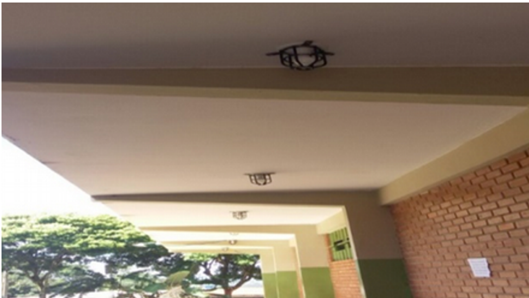
Photograph 3. Lighting system located in the corridor of the classroom block, after the intervention.
