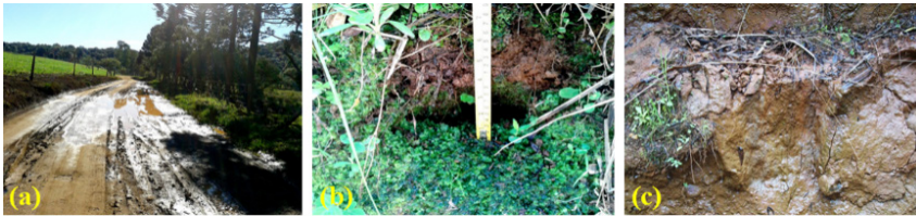
Figure 3- Identification of potential areas for interception of subsurface flow by rural roads. In (a) saturated area, in (b) active pipe, in (c) water exfiltrated on the embankment of the road
